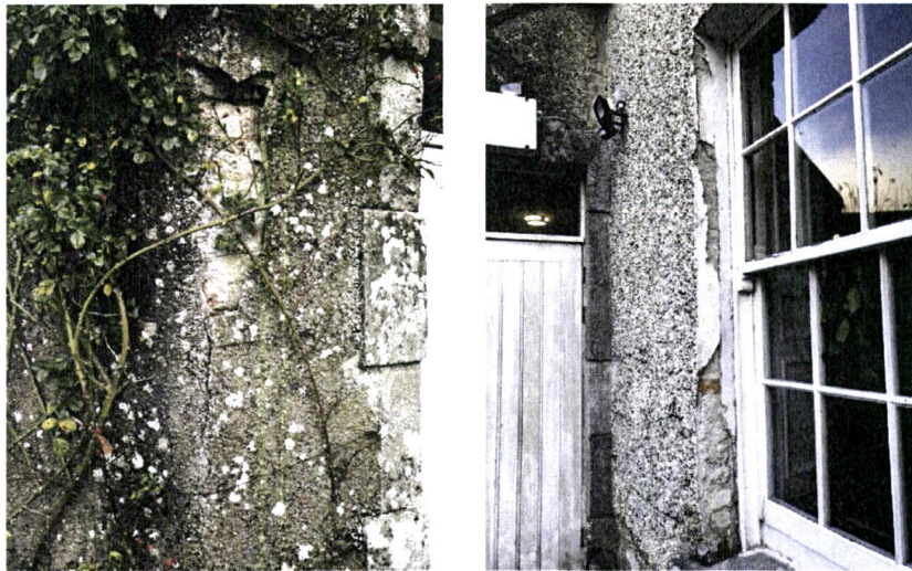
Close-up of privy wall (south elev) Examples of loss of material and delamination to a. door stone surround b. window reveal
